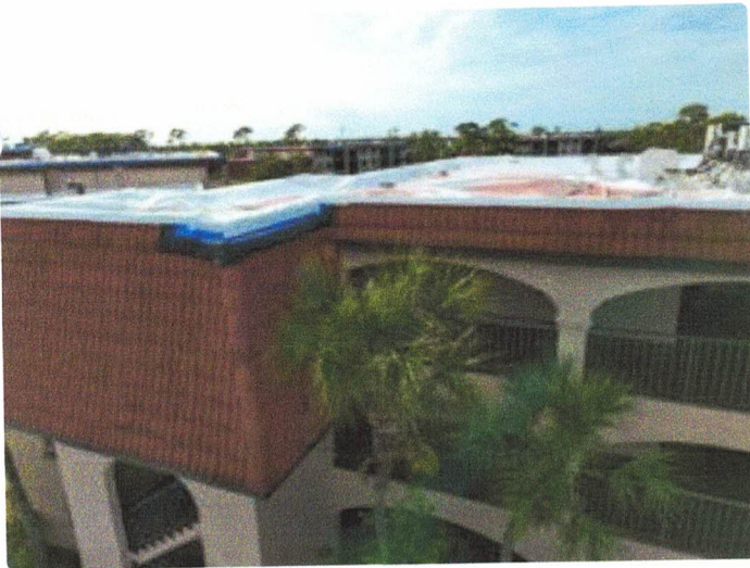
Broken barrel tiles
