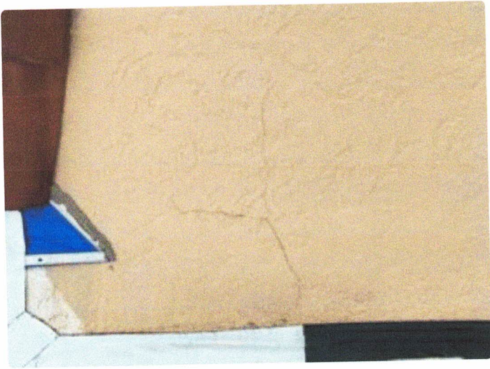
Crack on side of building on roof
