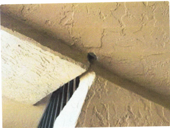
Crack under stairwell
