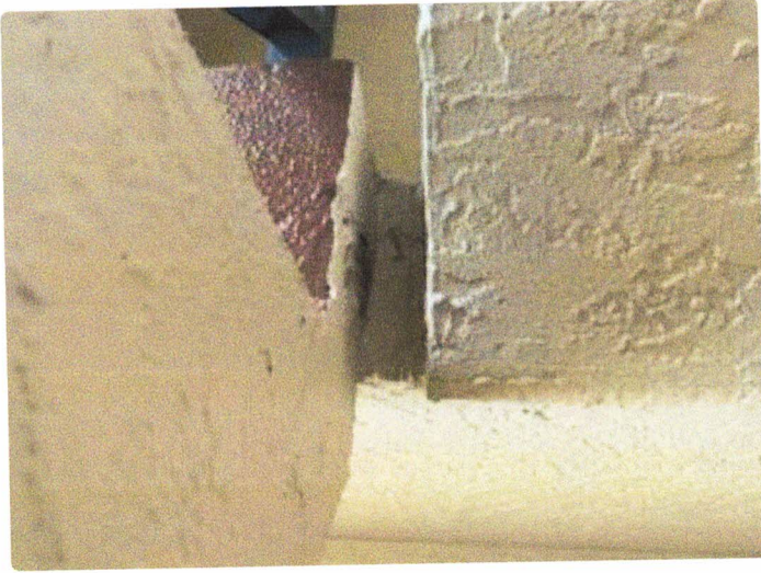
Spalling on right stairwell landing
