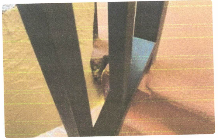
Spalling on landing
