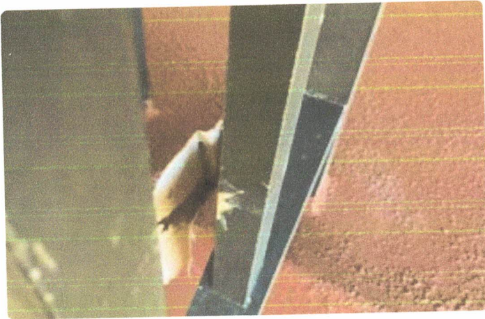
Spalling on face of landing
