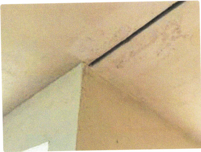
Gap in control joint under walkway
