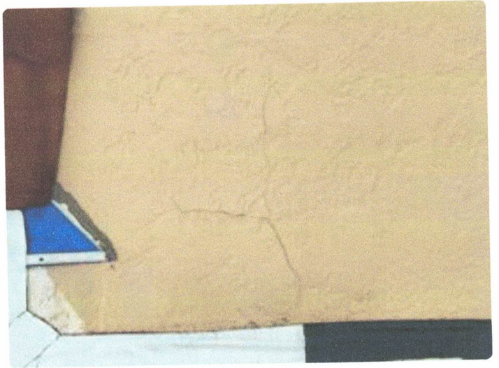
Crack in exterior wall on roof
