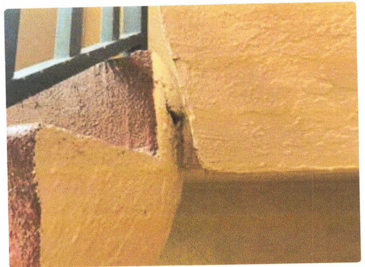
Spalling on right stairwell landing
