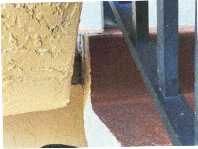
Spalling on left stairwell landing
