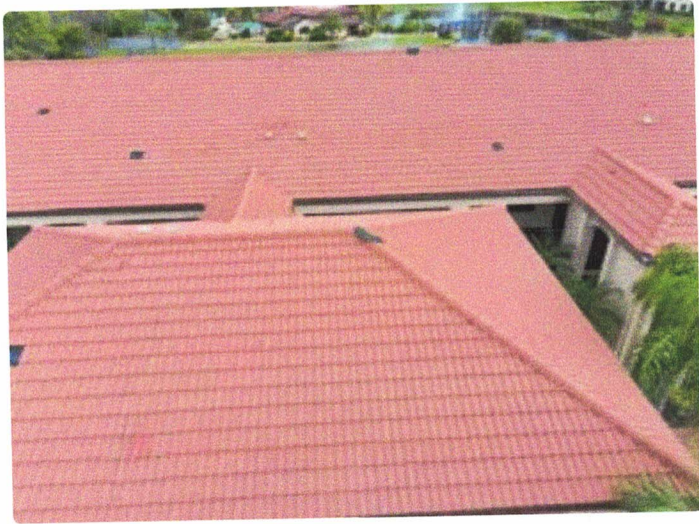
Broken barrel tiles
