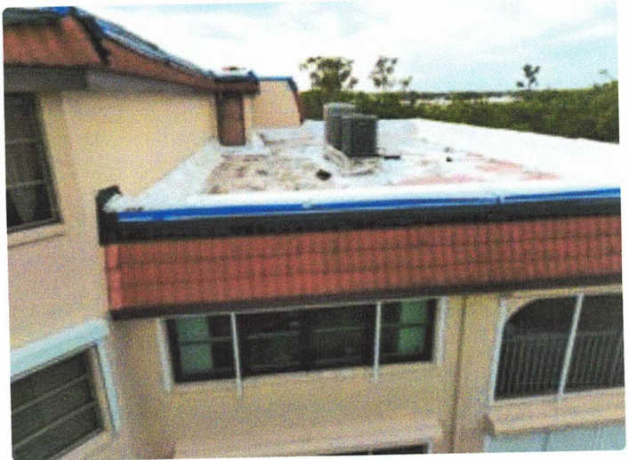
Gap at tiles
