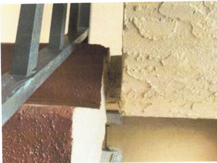
Spalling on right stairwell landing
