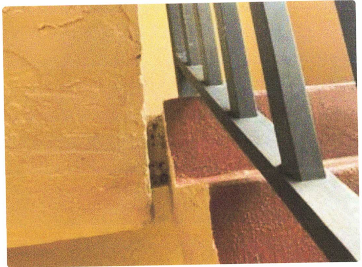
Spalling on left stairwell landing
