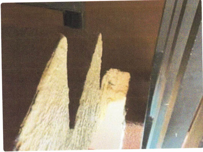
Spalling on left stairwell landing
