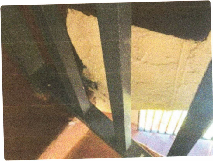
Spalling inside stairwell
