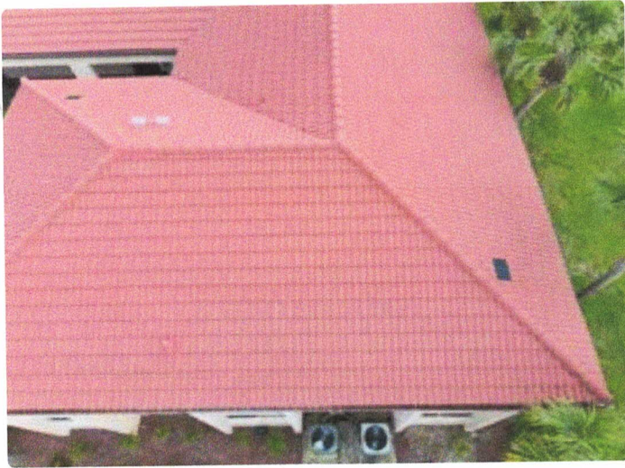
Slipped barrel tiles
