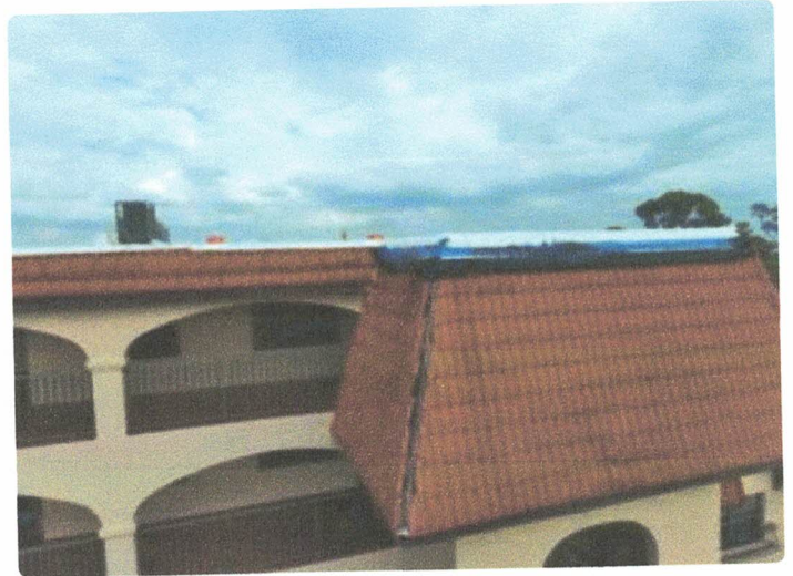
Broken barrel tiles
