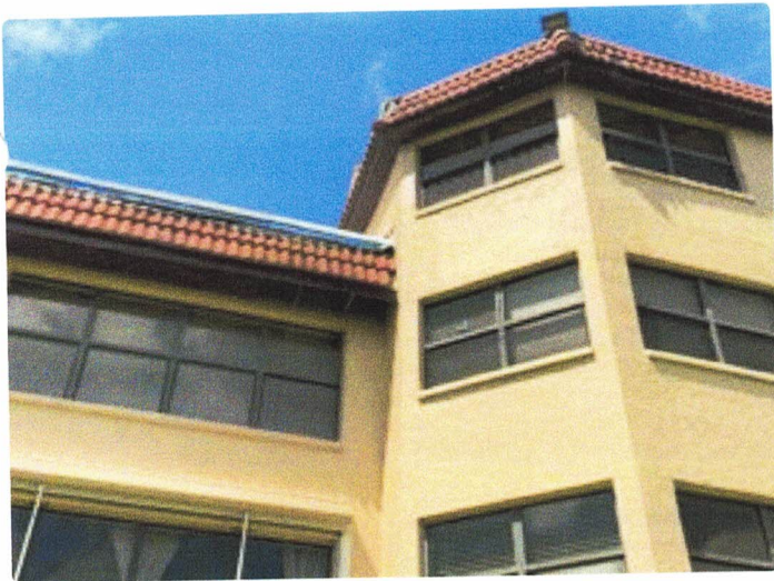
Broken barrel tiles
