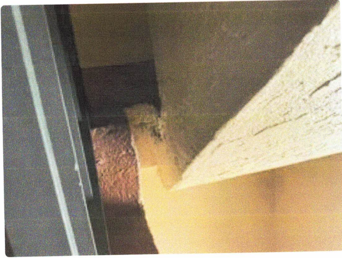
Spalling on right stairwell landing
