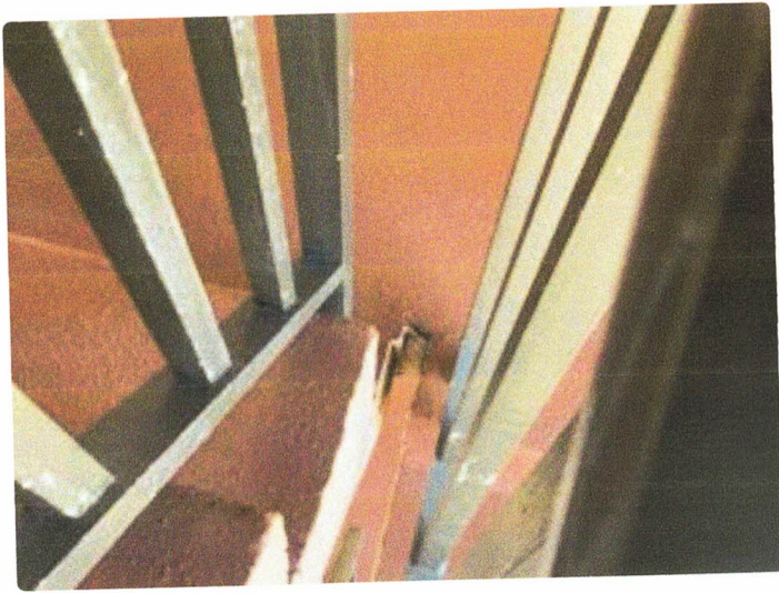
Spalling at landing on stairway
