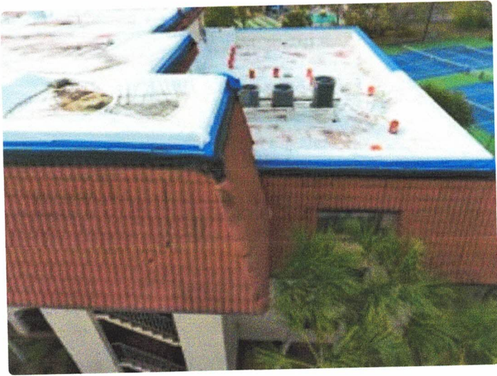
Broken barrel tiles
