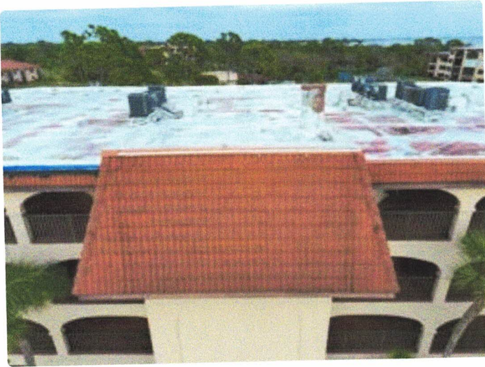
Broken barrel tiles
