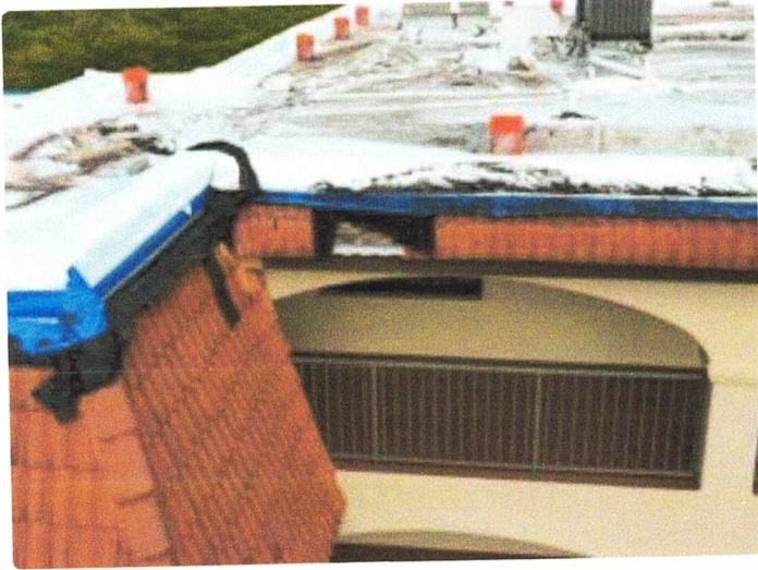
Temporary remediation failure
