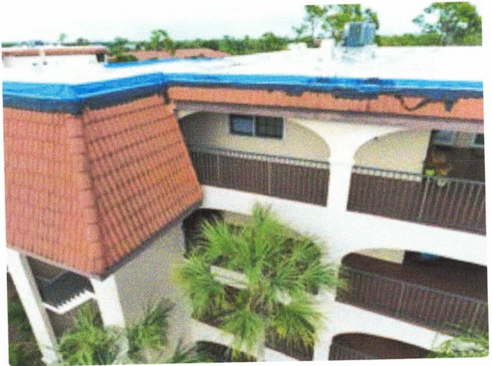
Temporary remediation failure
