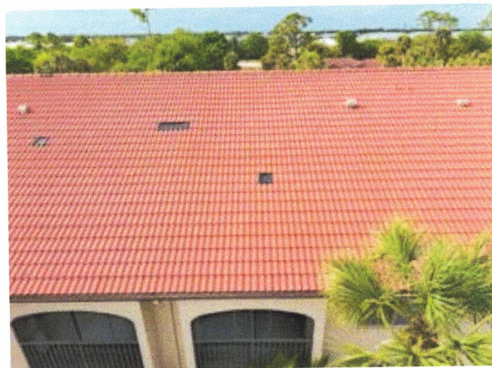
Broken barrel tiles
