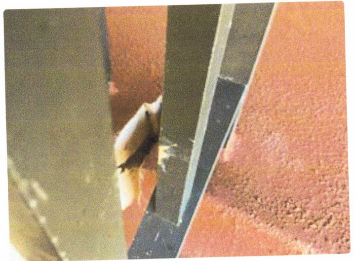
Spalling at landing on stairway
