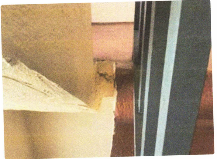
Spalling on left stairwell landing
