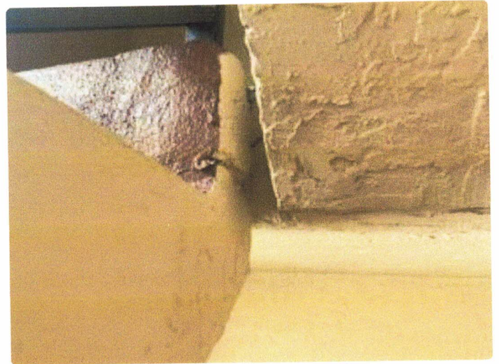
Spalling on right stairwell landing
