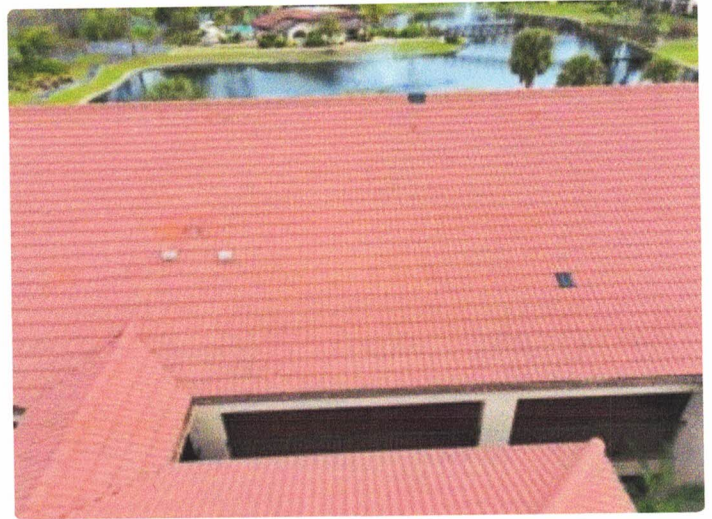
Broken barrel tiles
