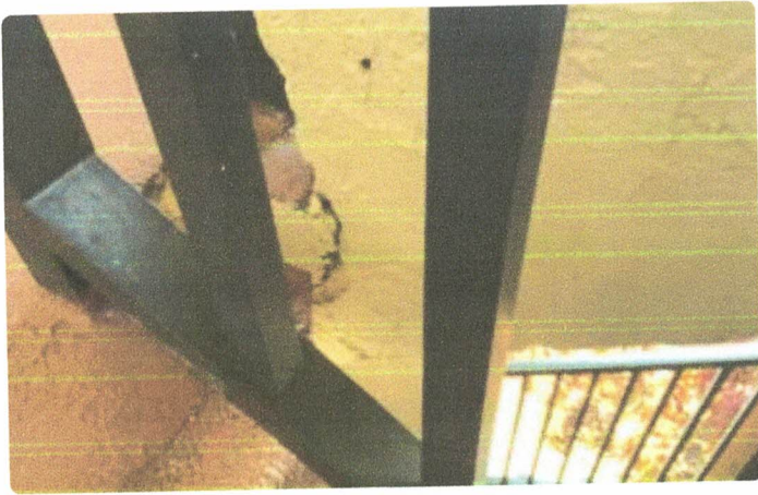
Spalling on landing
