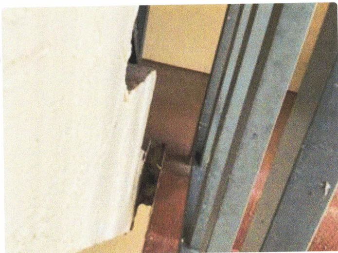
Spalling on left stairwell landing
