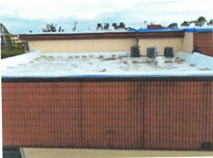
Broken barrel tiles
