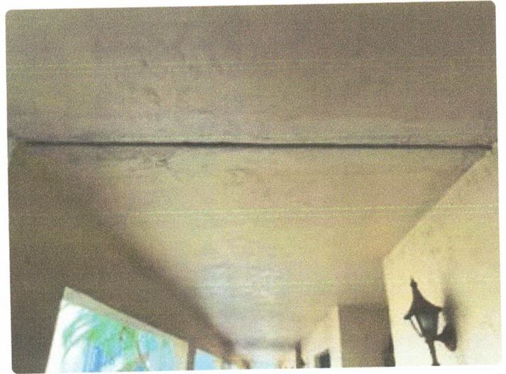
Gap in control joint under veranda walkway
