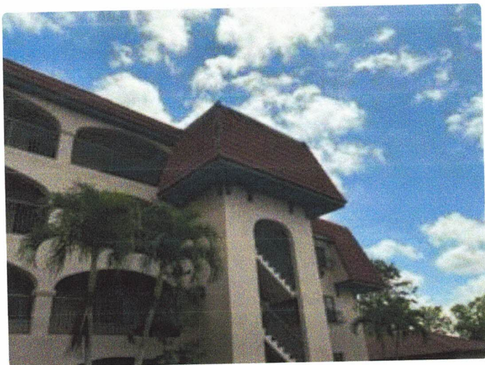
Broken barrel tiles
