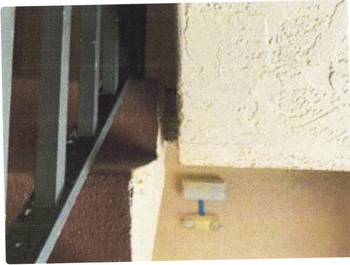
Spalling on right stairwell landing
