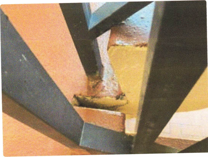
Spalling on inside of stairwell
