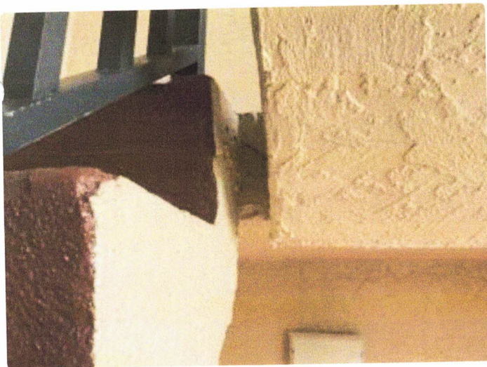
Spalling on right stairwell landing
