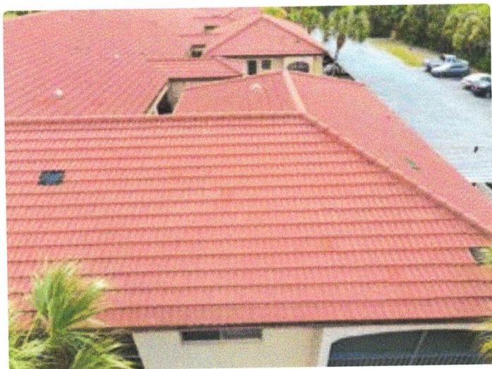
Broken barrel tiles
