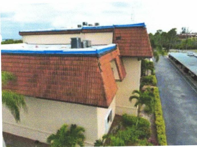
Broken barrel tiles
