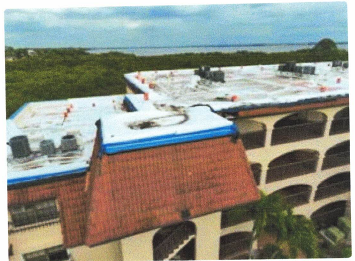
Broken barrel tiles
