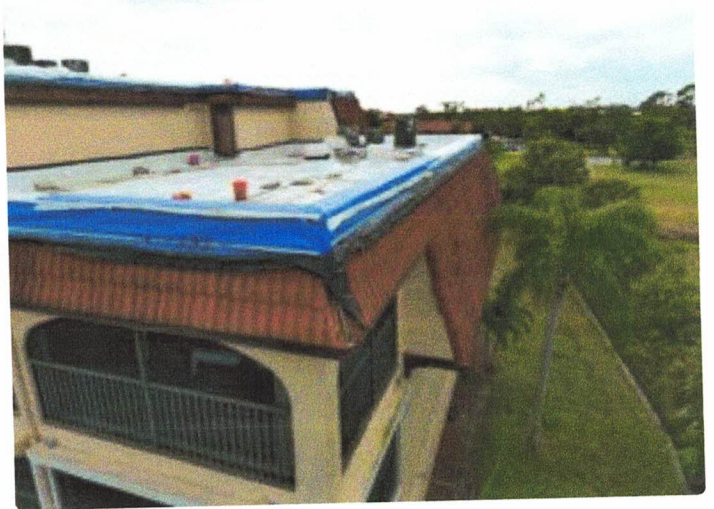
Broken barrel tiles
