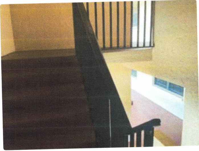
Loose railing cover
