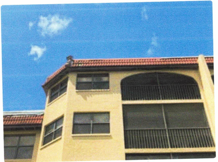
Broken barrel tiles
