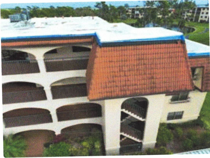
Broken barrel tile
