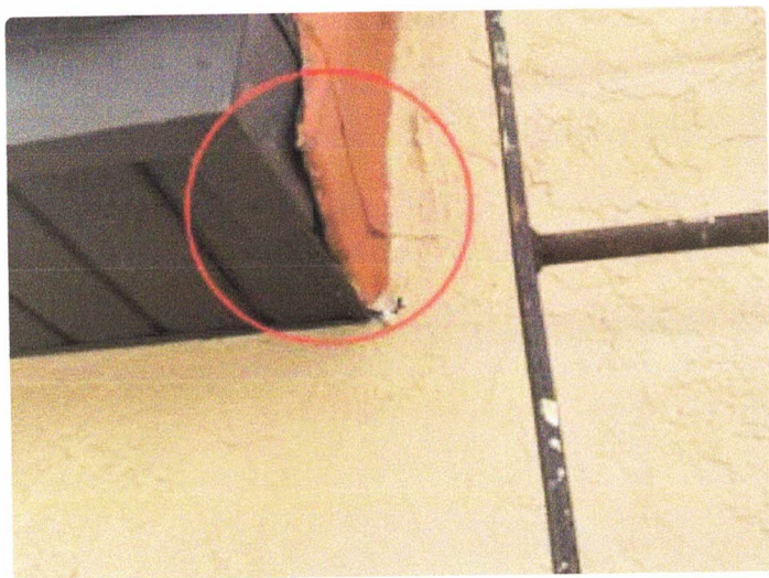
Gap at flashing
