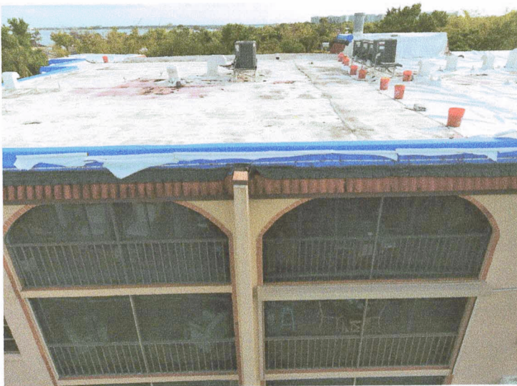
Partially tarped roof post lan
