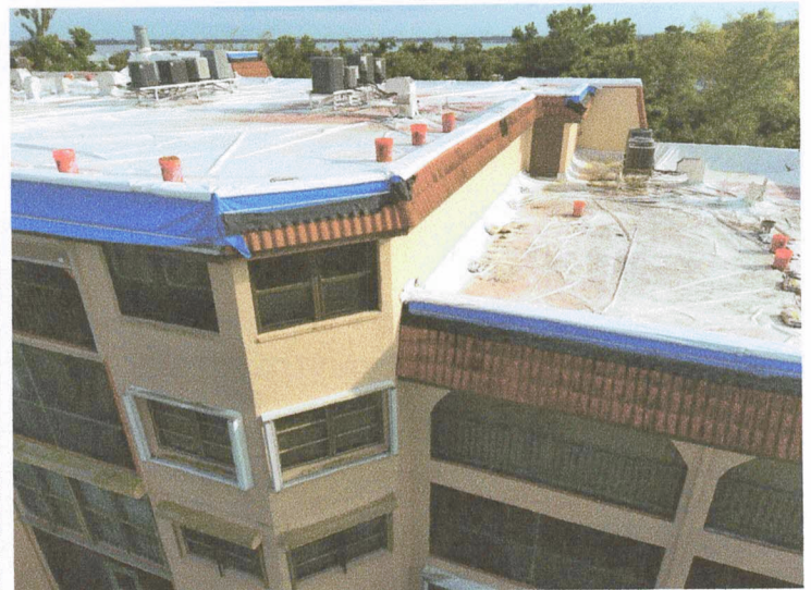
Tarped roof post lan
