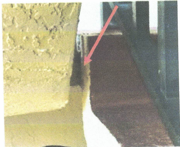
Gap at top of stair landing
