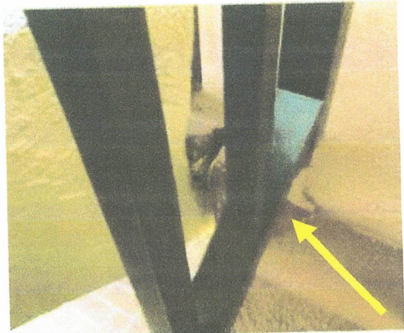
Spalling at top of stair landing
