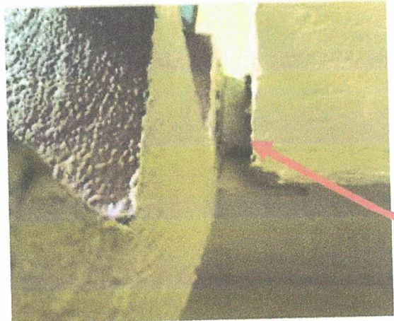
Gap at top of stair landing
