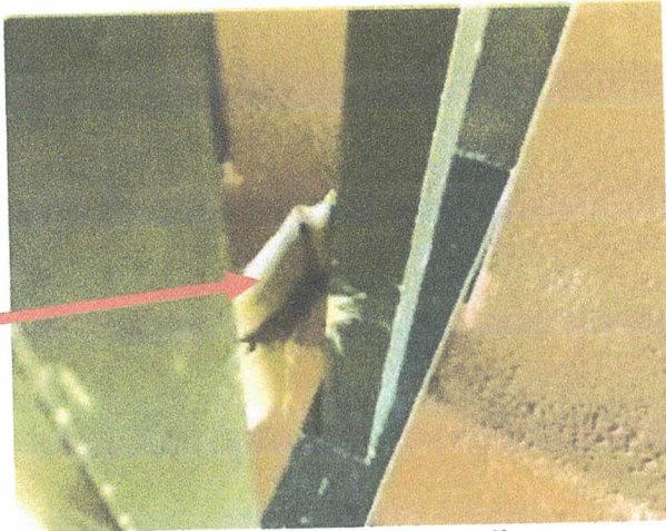
Gap at top of stair landing
