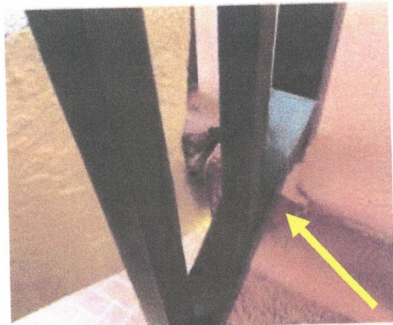
Spalling at top of stair landing
