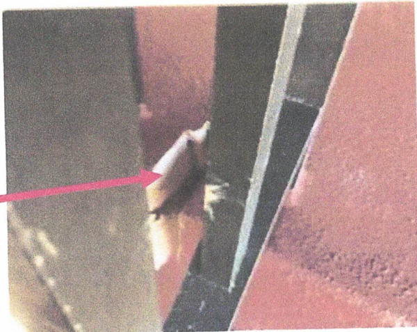
Gap at top of stair landing
